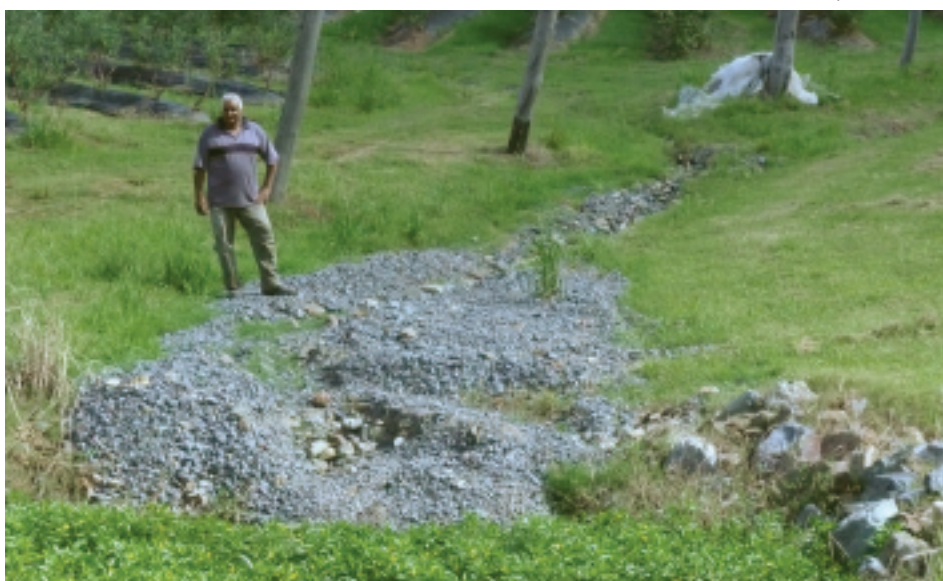
Subsurface drainage improves the central flow line
