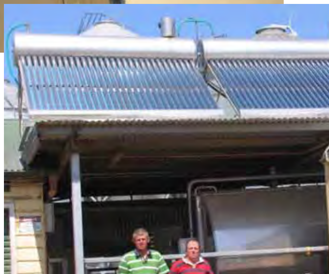
Top: 2 panels have 250 litre tanks on the roof, the third recirculates to a tank in the dairy.
