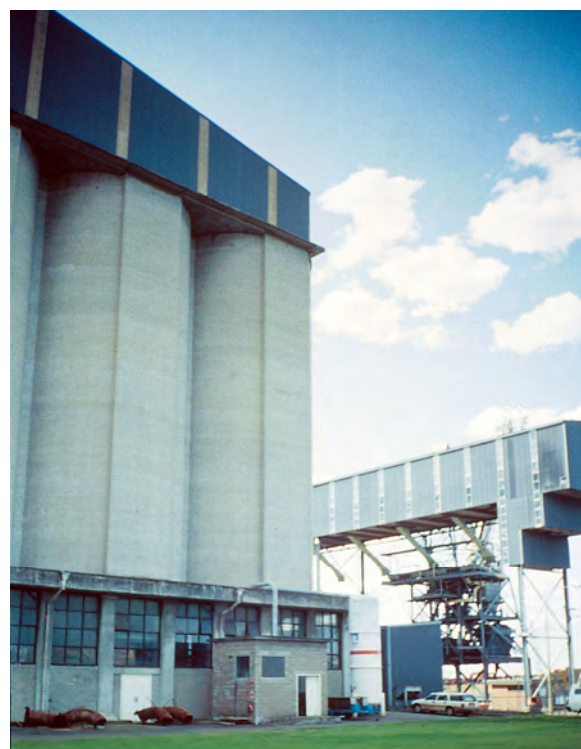
Figure 3. Bins at Newcastle (NSW) export terminal under nitrogen disinfestation treatment before export. The nitrogen storage is at the base of the bins. Photo Julie Cassells (© CSIRO).
